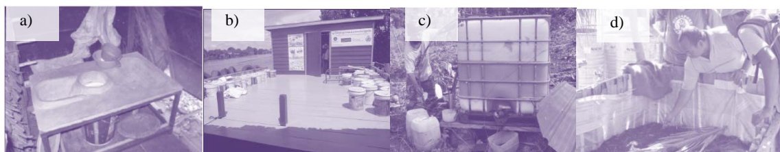
Figure 4 a) Dry and separated toilet with container; b) Waste collection station; c) Urine container; d) Composting site (Brown, 2010; Sayre et al., 2011)
