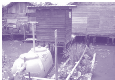
Figure 3 Application Compact Biofiltration System in Banjarmasin (Sumidjan, 2012)
